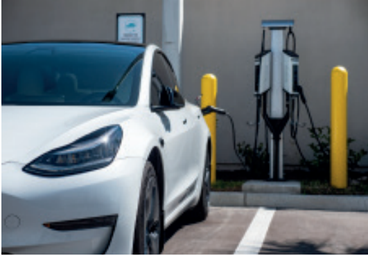
SemaConnect's open network has made EV charging stations accessible to more than 1 million EV drivers in the U.S.
